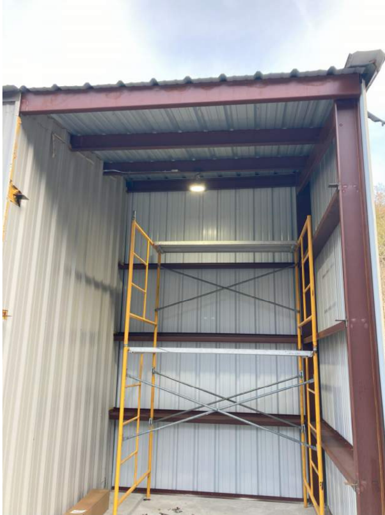
Figure 10: Building add on for temperature controlled chemical storage
