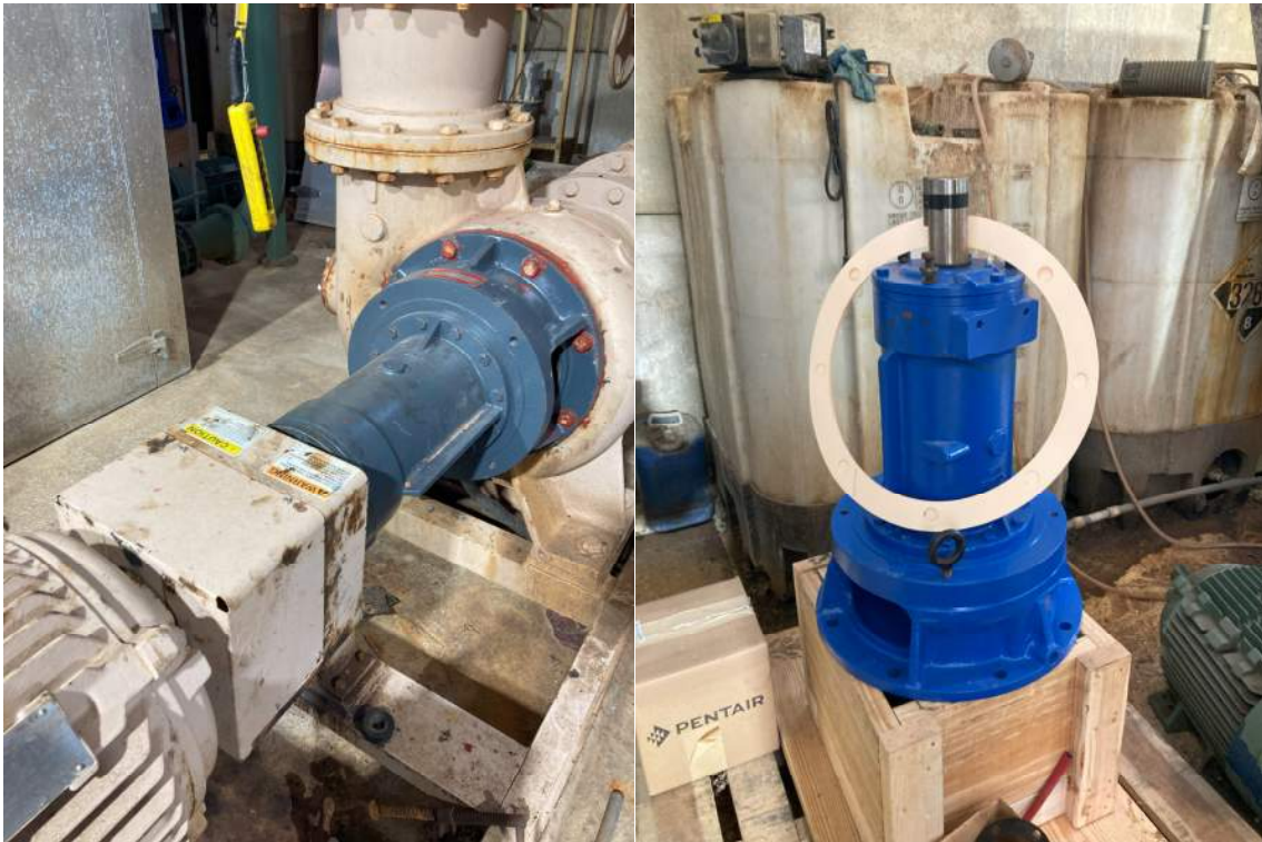
Figure 6: Rebuilt motive pump for SBR#1 in service (left); new backup pump (right)
