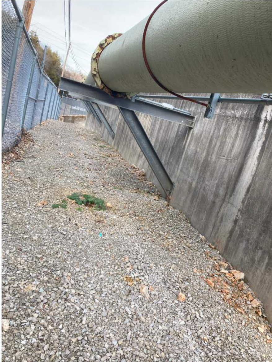
Figure 1: West side of SBR system where initial overflow occurred indicating there have been no recent overflows
