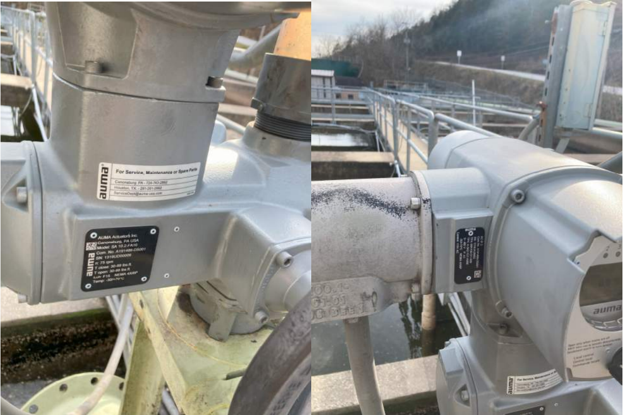
Figure 7: Influent valve for SBR#1 in operation
