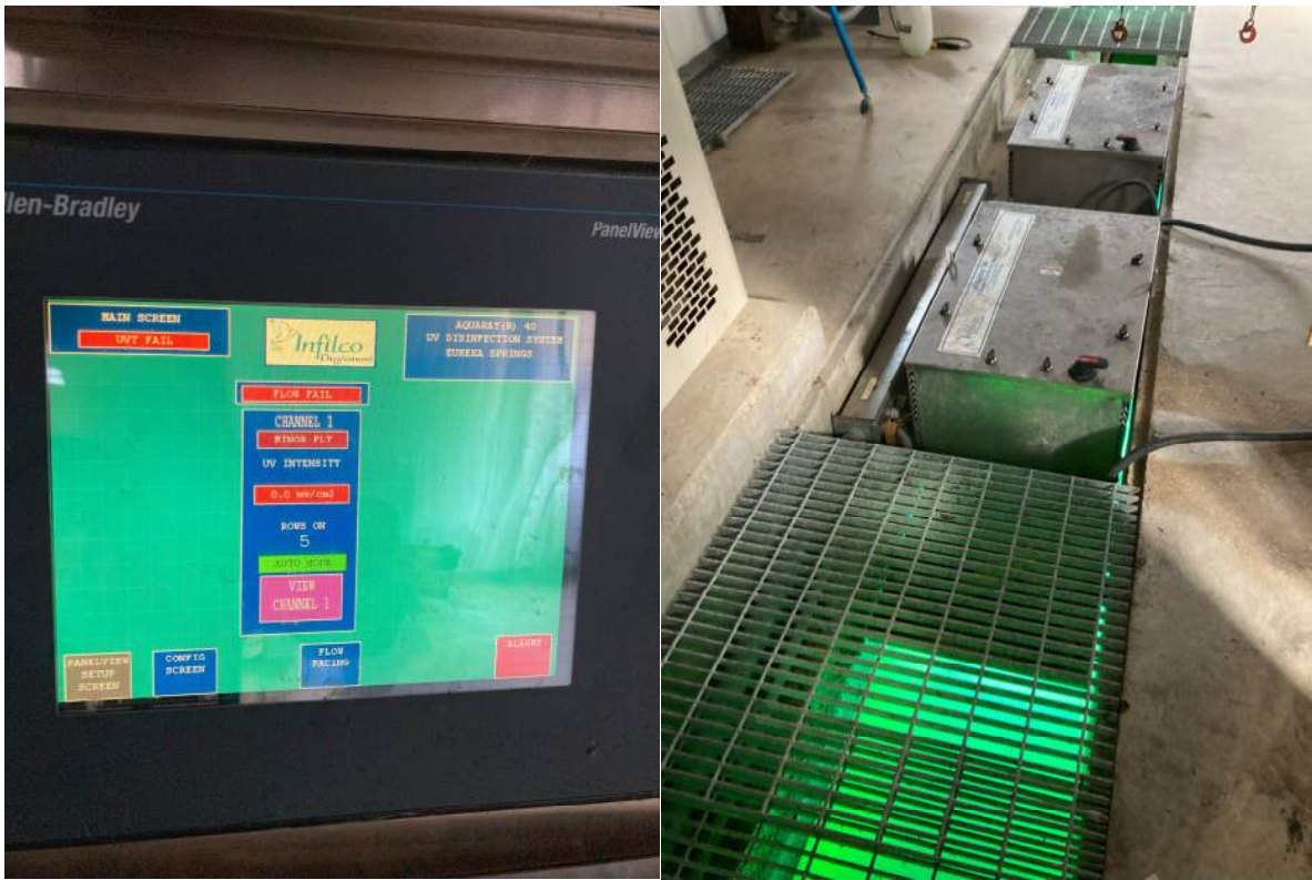
Figure 8: Ongoing issue with communication (left); both UV modules in operation (right)
