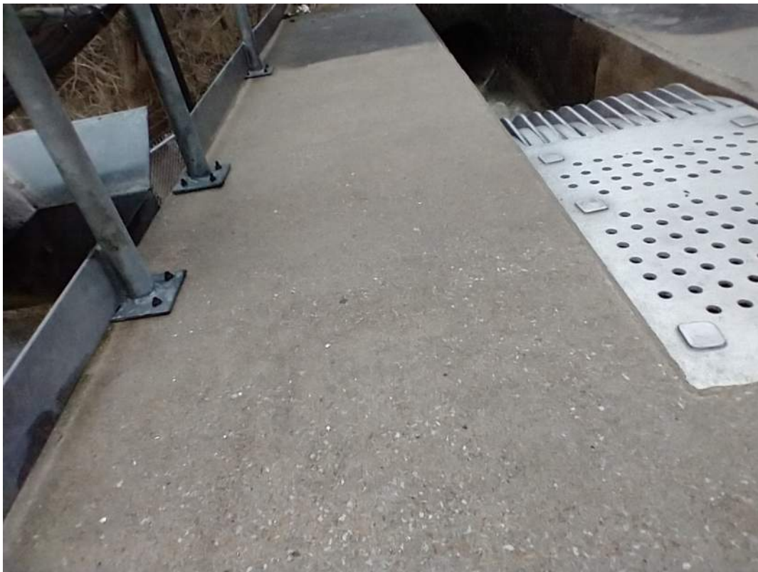
Figure 2: Concrete slab adjacent to slab after cleaning
