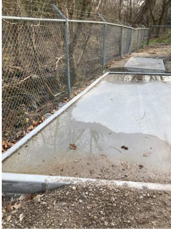
Figure 3: East side of newly constructed concrete slab adjacent to screening and grit removal equipment.
