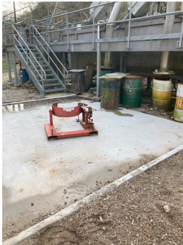
Figure 4: West side of newly constructed concrete slab adjacent to screening and grit removal equipment.
