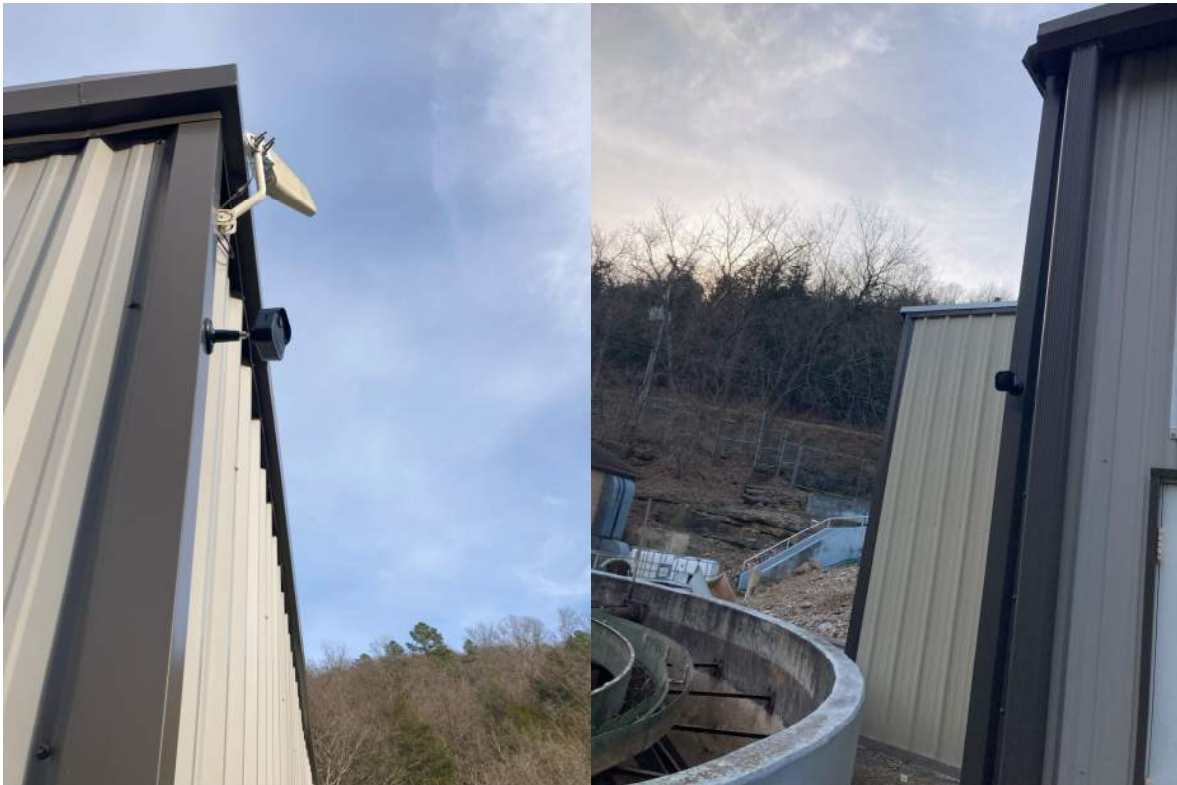
Figure 9: Camera used to monitor SBR basins (left); camera to monitor fence gap and sludge storage (right)
